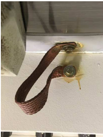
Figure 7: loose earthing strip
