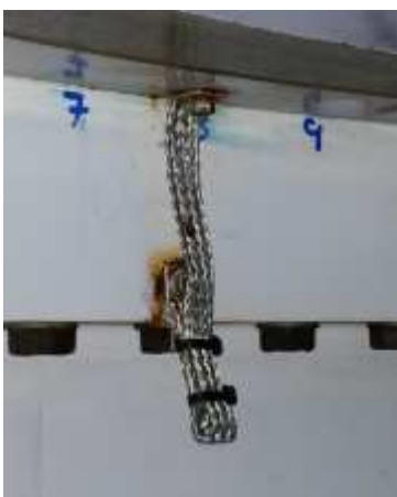
Figure 9: earthing strip going down in the magnet area.
