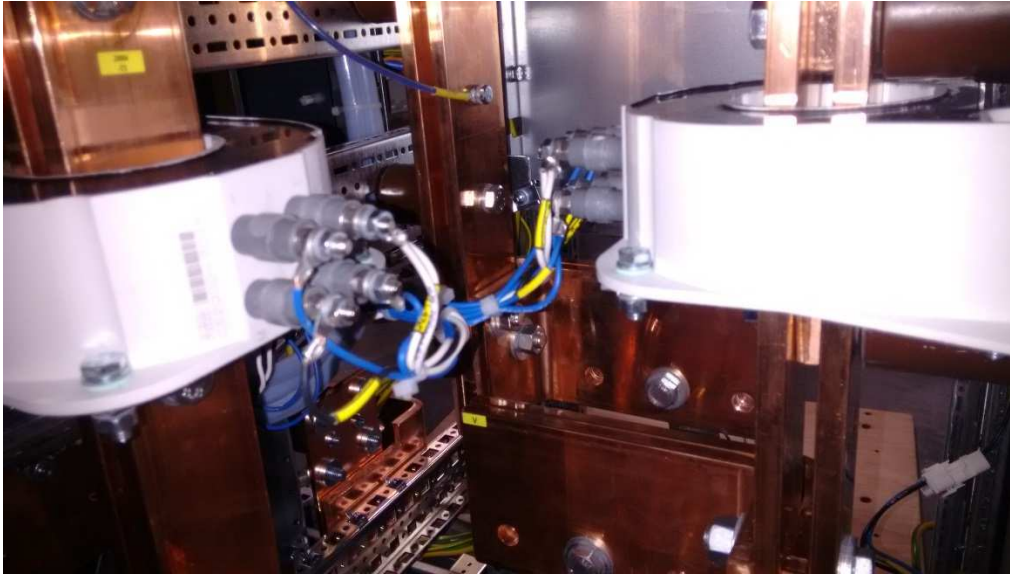
Figure 28: Transducer at busbar of stator circuit in the incoming feeding unit +1S3 of ProWind IV with dis-mantled back wall left in this picture: transducer phase U D004-T3, right in this picture: transducer phase V D004-T4, middle rear: phase W busbar without transducer
